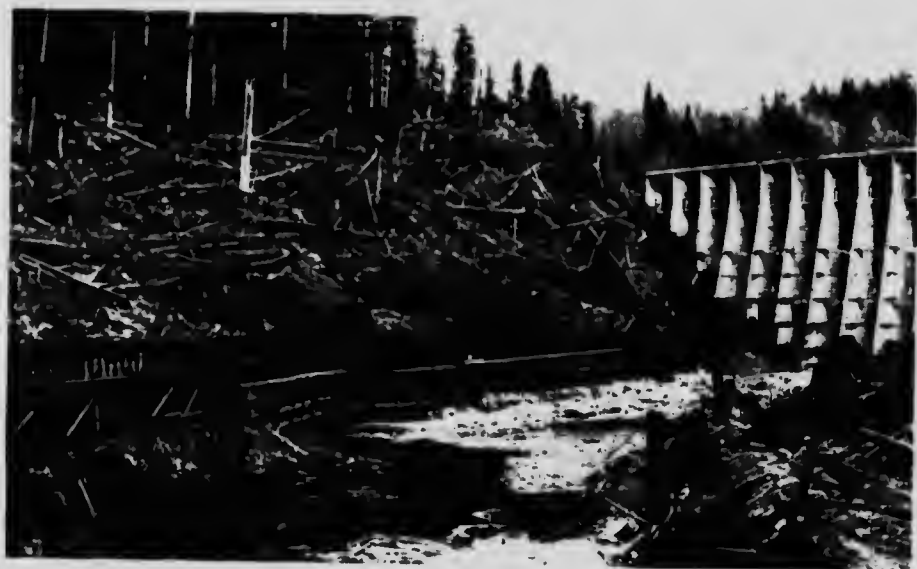
Vancouver Island Power Company Limited. Jordan River Dam. Crib work for protection of new flume below Dam.
